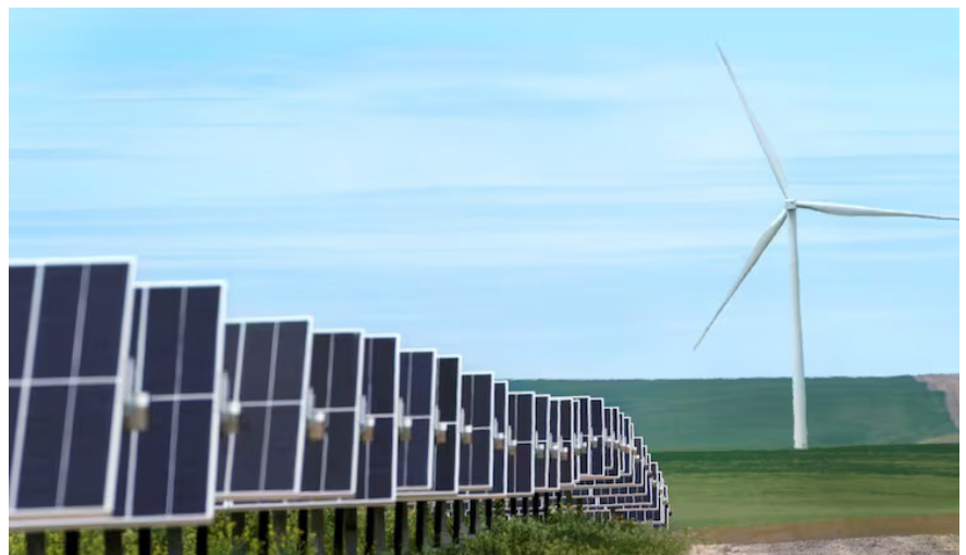
Portland General Electric has teamed with NextEra Energy Resources to build a ground-breaking, first-of-its-kind facility that can store solar- and wind-generated electricity. It uses an innovative battery technology that has been called a game changer.
