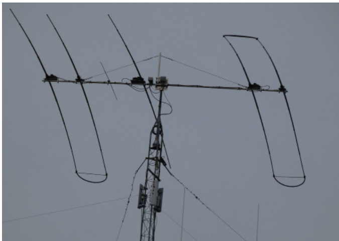
Two large AREDN antennae installed below WV ham antenna.
